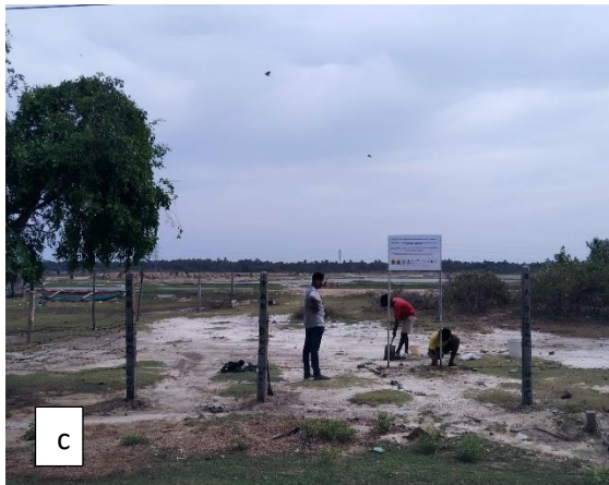
Figures 23: (a) The officials from DWC & DAD with the project team, after examining the site for clearance, (b) DAD officers securing the reservation boundary of the tank, (c) Initial site preparation, August 2022
