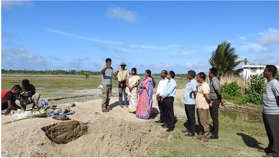
Figure 24: Ceremonial foundation laying of the birdwatching blind with the participation of stakeholders, October 2022
