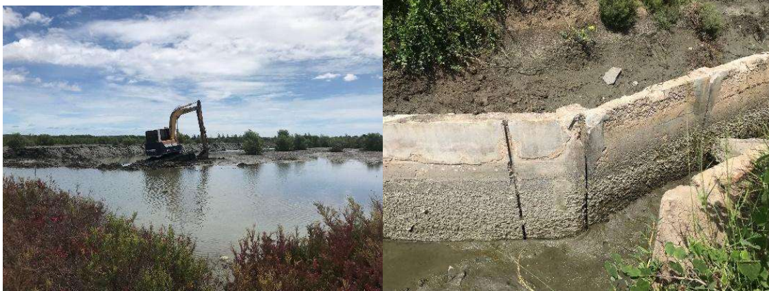
Figure 2. Habitat and water management for shorebirds. Works to create soil bunds and mounds and the construction of a water drainage system in Pak Thale's salt pans.
